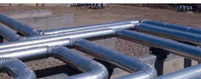
Extensive pipe system's
